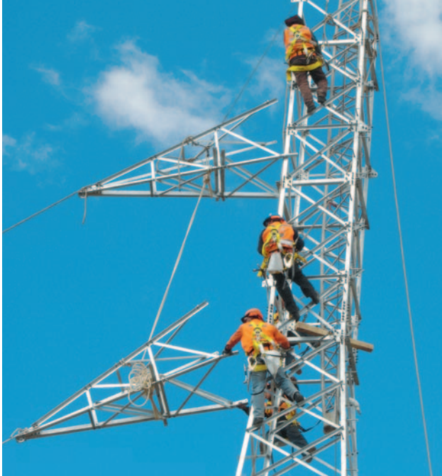
Safety training, procedures and equipment make for safe work on the 100-kilometer power line supplying energy to Lagunas Norte (Peru).
