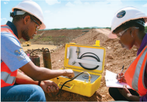
Environmental staff monitor pore pressure on the water storage dam wall at Tulawaka, our newest mine in Tanzania.
