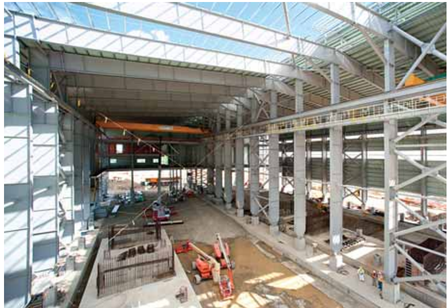
Large scale autoclaving of gold, pioneered by Barrick at Goldstrike, is being constructed at the Pueblo Viejo project in the Dominican Republic.
