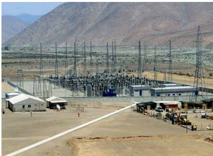
The primary substation at Punta Colorada, Chile connecting to the main power grid from which Pascua-Lama will obtain its electrical energy.
