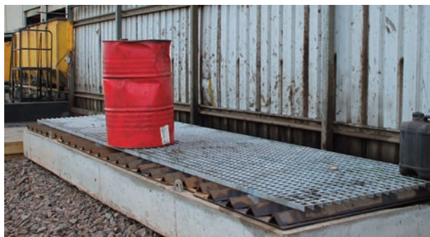
Osborne: Storage bunds for oil and fuel drums ensure containment.
